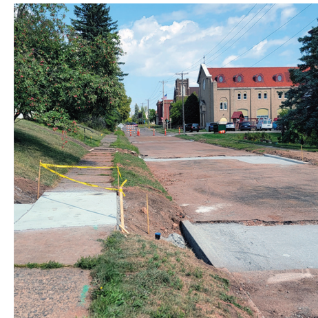
Duluth is one of many Minnesota communities that is replacing lead pipe service lines.
